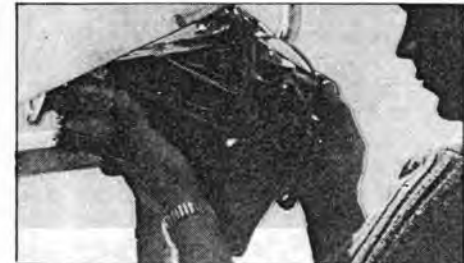
Fitting the differential unit. This has to be fitted from the nearside and if the diff brace is fitted (Sprint) then remove it and fit on after the diff is in. It is a very tight squeeze to get it in - a block of wood and hammer sometimes helps!
