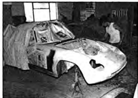
Localised spray of I.C.I. spray filler over the join and gel crack areas. Although the new section comes ready in primer-surfacer from the factory, we virtually flat it all off and start again. The photograph may not show this too well.
